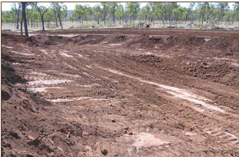
PHOTO 9: Push subsoil into gully and reshape with low profile batters. Construct the diversion bank around the gully head.
