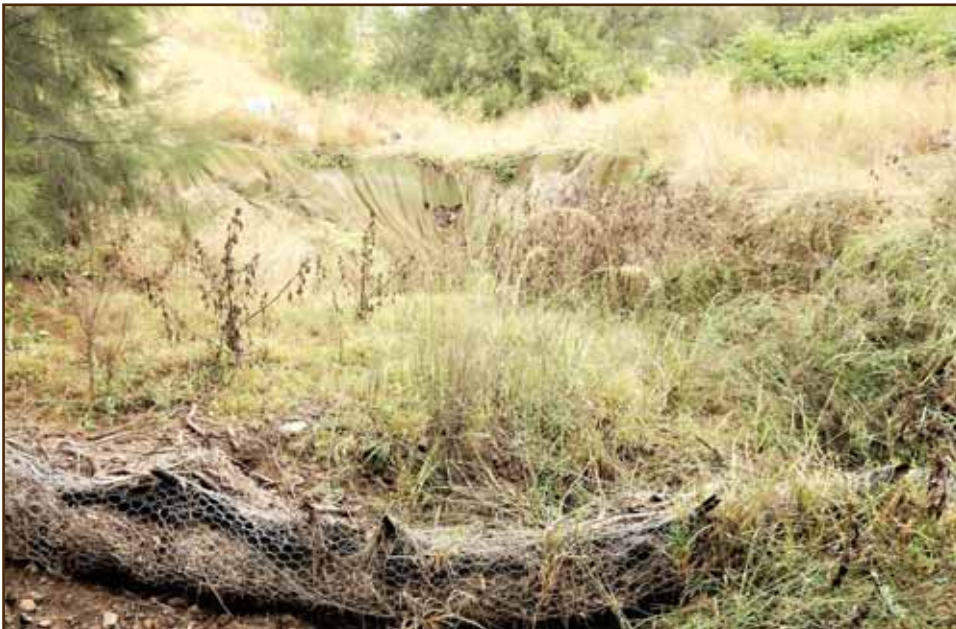
SITE 1 PHOTO 62: After two years of rainfall events, good grass cover is evident on and around the structure. The damage to the geofabric that can be seen in this photo was repaired.
